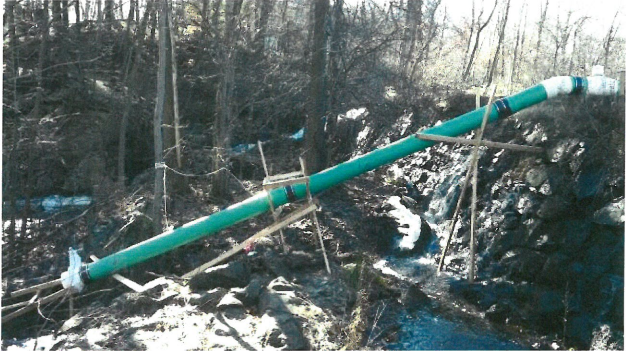
Photo 3: Front of Dam (Seepage through face of dam. Temporary piping installed to drawdown water level of the dam.
